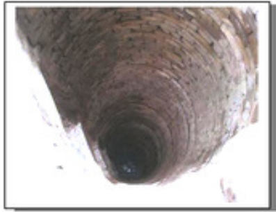
Abandoned Dug Well
